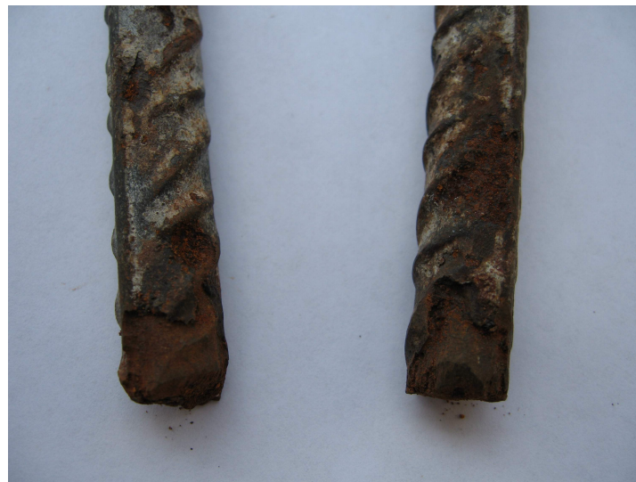
Fig. 13. Heavy corroded reinforcement in concrete made with Type V Portland cement after 4 years
