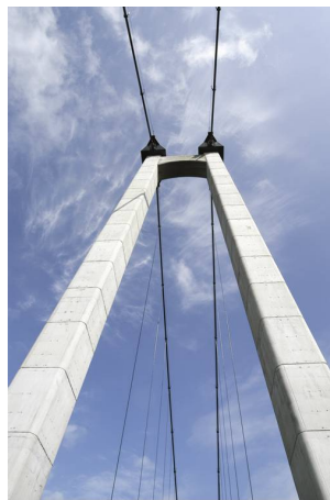
Fig. 1b: Concrete Bridge, which was produced with CEM II/A-V concrete in Scandinavia in the year 2001. The bridge shows no scaling or cracks.
