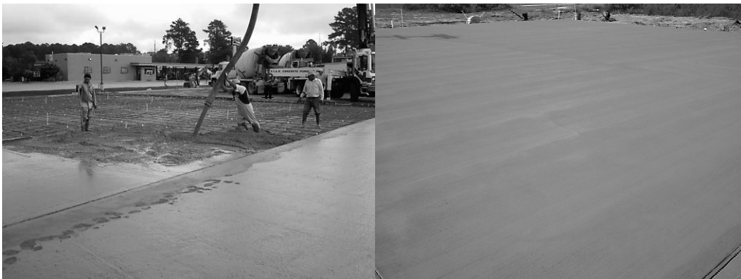
Fig. 2. Pouring concrete for the truck stop (left) and concrete surface of the truck stop after setting (right).
